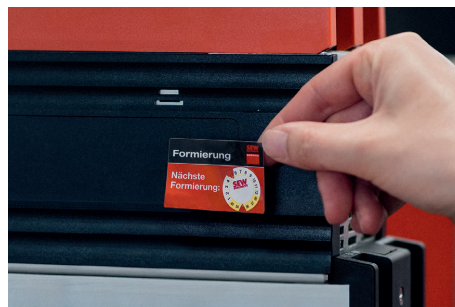
Labeling of checked frequency inverters
